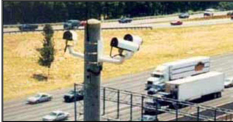
Figure 8: Video Detection System Cameras in Atlanta, GA (Source: http://www.georgia-navigator.com/about )
